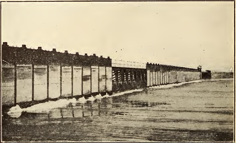
FIG. 29.—Gates in Milner Dam, Snake River, Idaho. At times of high water these gates are raised to regulate flow in canals.
